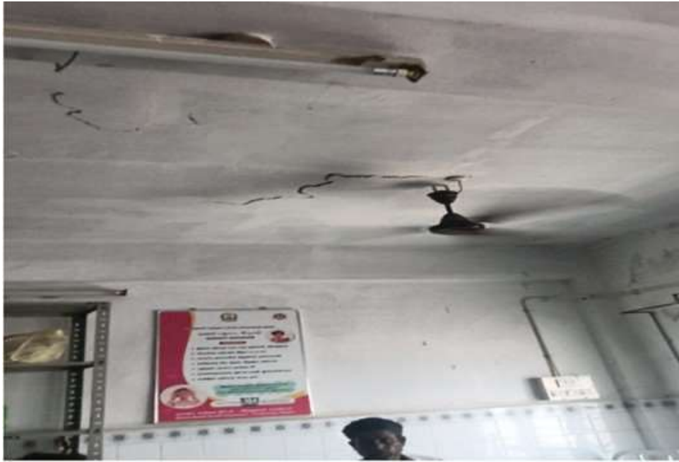
Figure 3.9: Cracking ceiling in the male ward old block of an accredited GH, with risks to patient safety
