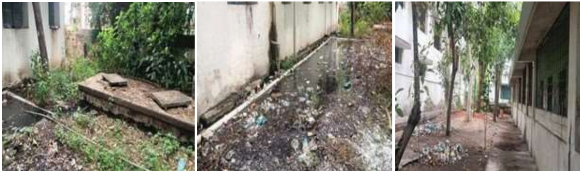
Figure 3.5: Backside of the old block with sewage water stagnation and landscaping of an accredited DH
