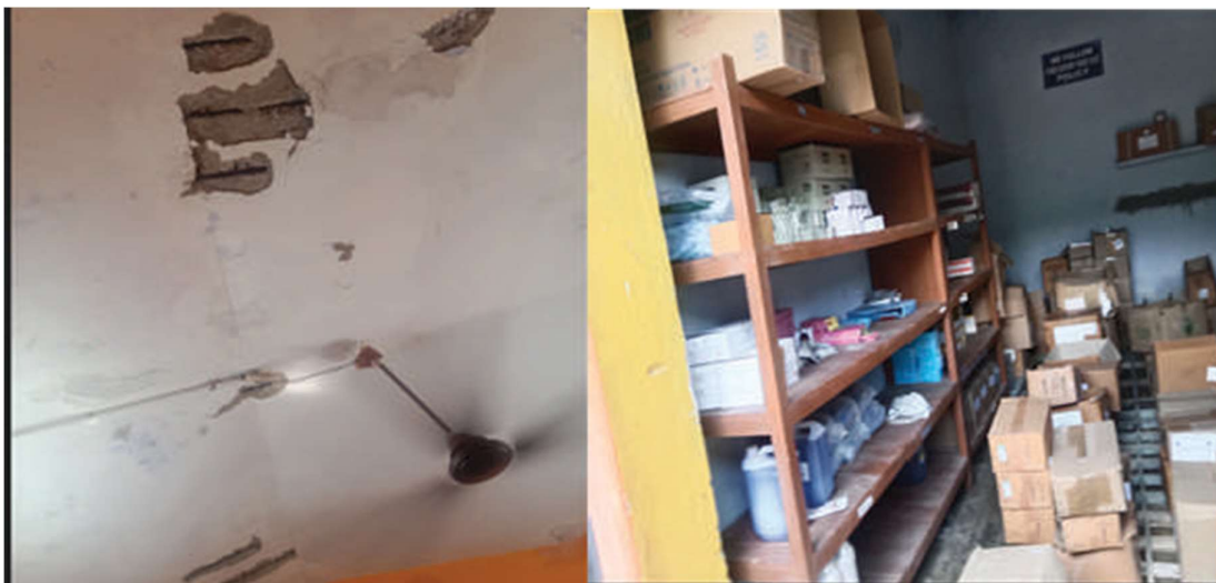
Figure 3.10a: Roof falling apart in the pharmacy counter room where tablets are issued. Figure 3.10b Ambulance garage converted into pharmacy main store in an accredited primary facility.
