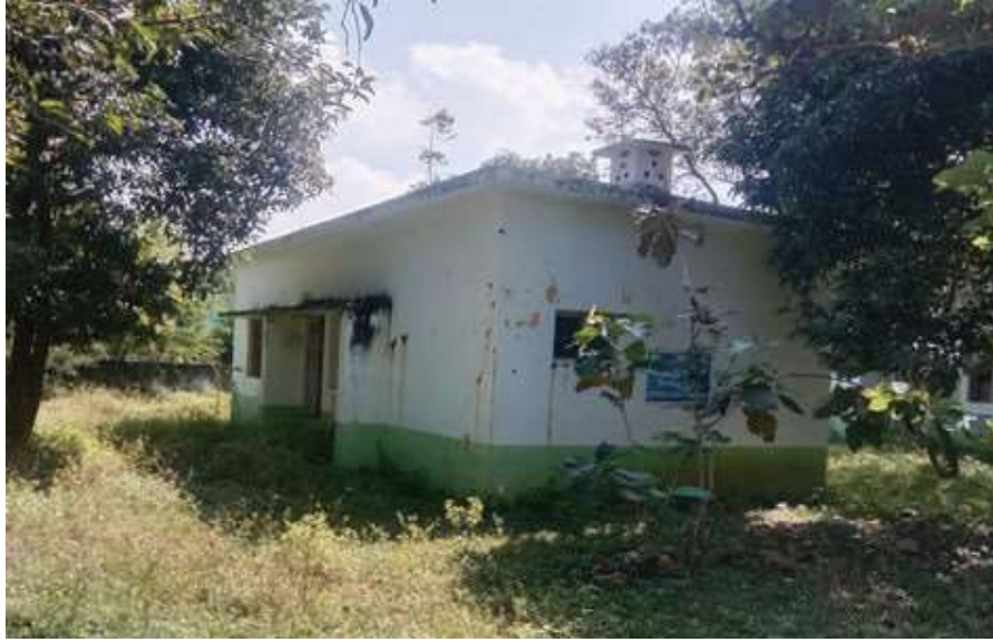
Figure 3.11: Condemned staff quarters used by ANM, Drivers and as BMW store room at an accredited primary facilities
